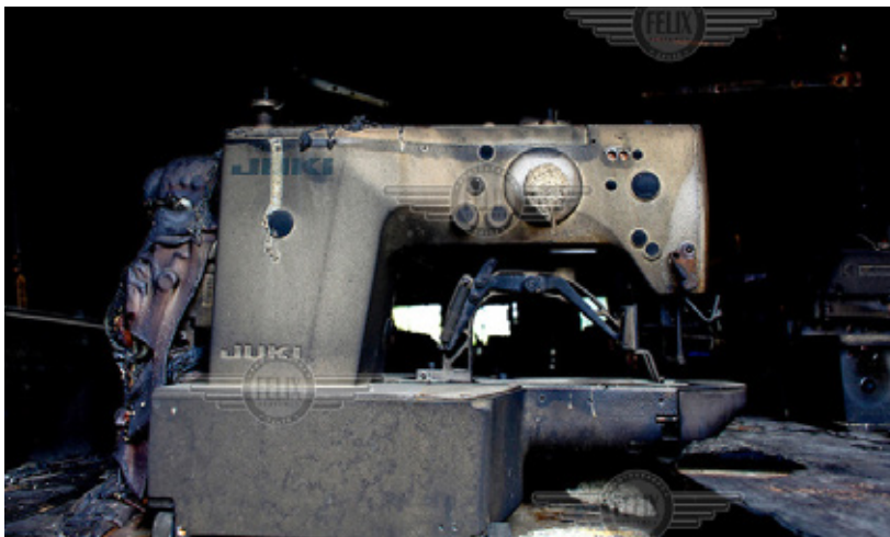
Damage to a sewing machine following the use of an oversized circuit breaker.
